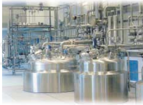
Large scale industrial multiple fermentor installation
