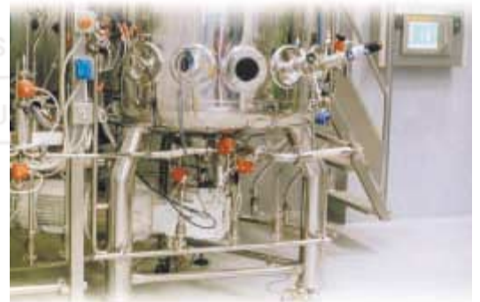
Fermentor control retrofit of an existing plant
